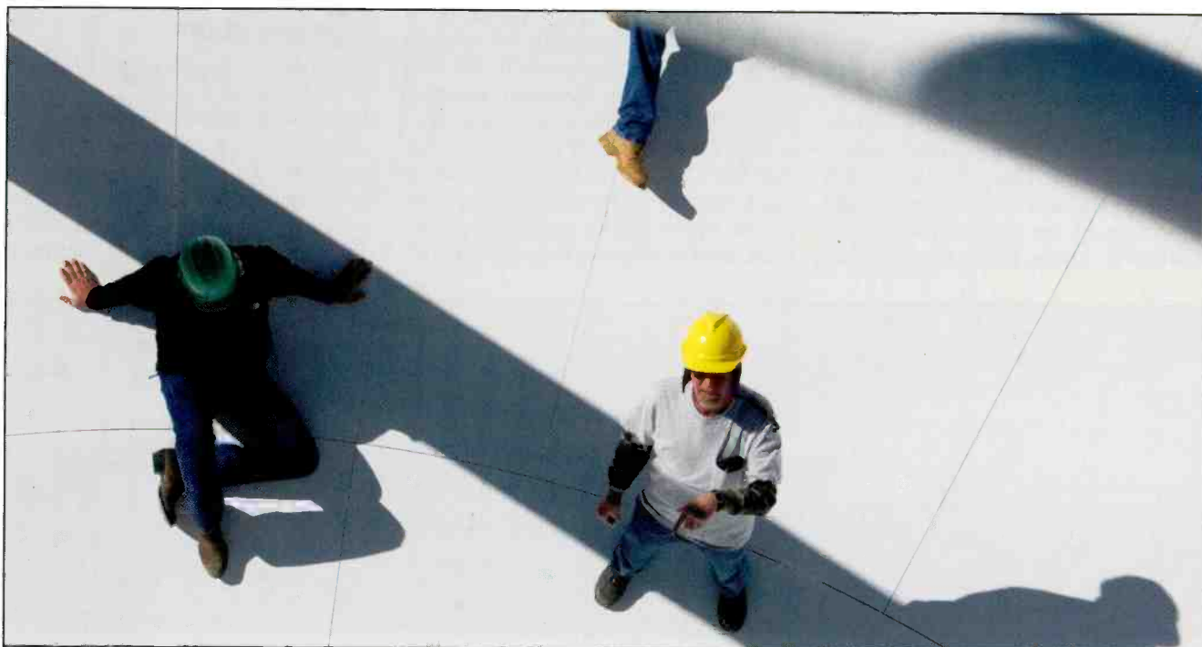
Photo N. "I can tell you, it gets dang hot inside that dish," writes NA5N, prompting workers to move into the precious-little shade there whenever possible.
