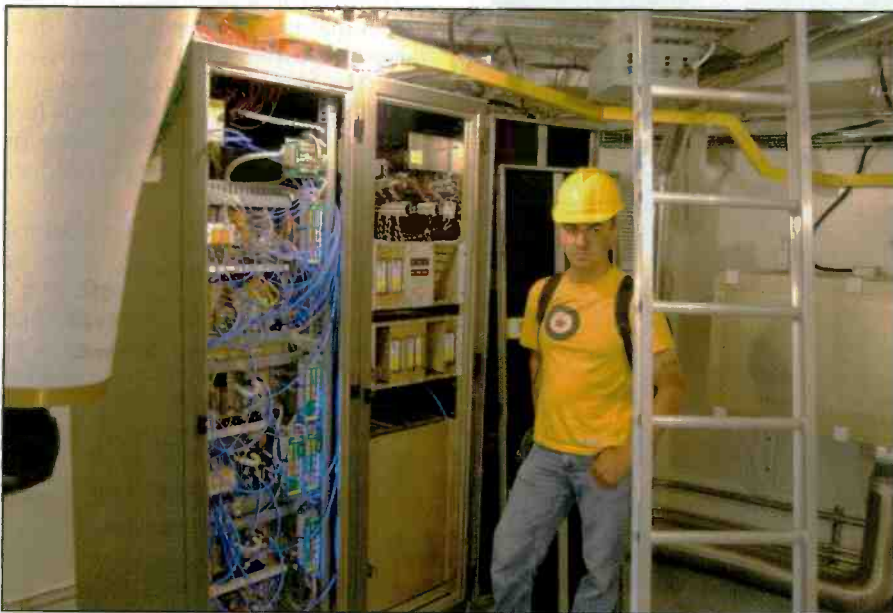
Photo F. Uncovered for the whole world to see is the LO/IF and front-end rack — just part of a mass of electronics required for VLA-supported research at NROA.
