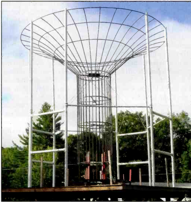
Photo D. Here's a picture of the CFA installed at the WGFP transmitter site. (WPC1CAT photo)
