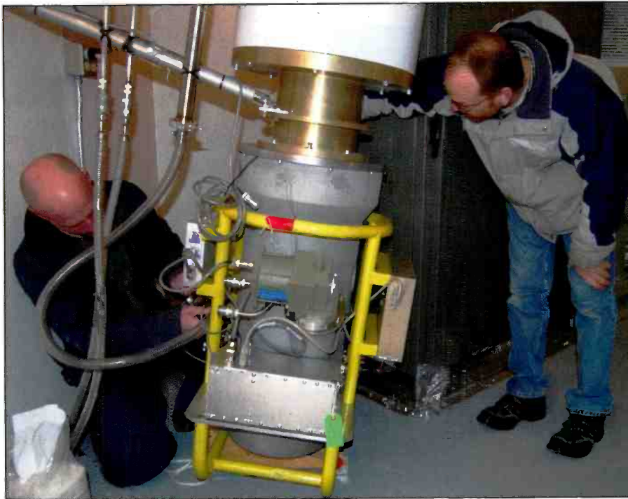
Photo H. Members of the VLA team connect the vacuum lines and the liquid helium cryo-lines. The unit operates at a near vacuum.
